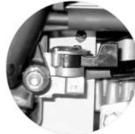
Fuel shutoff valve open.
