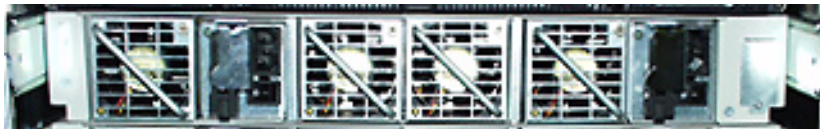
Rear View of 32-port Switch Installed in a 39U Rack
