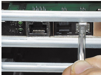
Standard phonenumber cabling with RJ-11 tips
