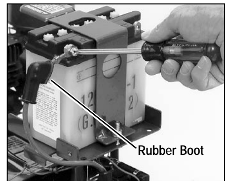
Figure 2-18: Attach positive (+) battery cable. Cover connection with rubber boot.
