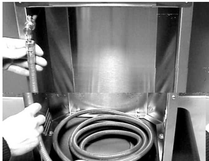
Figure 16 Natural Gas Hose Connection
