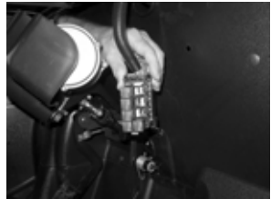
Step 3 - Cover removed
