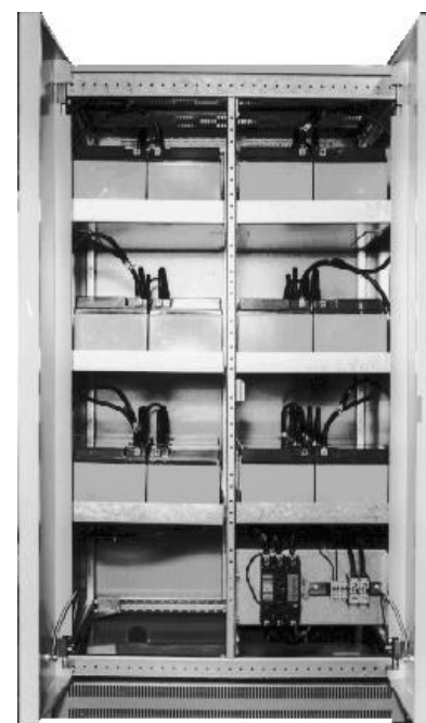
FIG. 1.12.4 Battery cabinet B3/38
