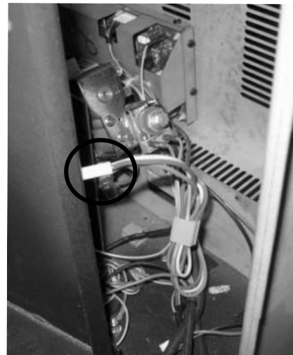
Wire Harness Disconnected
