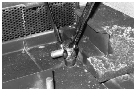
Burner Orifice Removal
