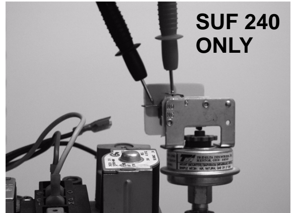
Low gas pressure switch
