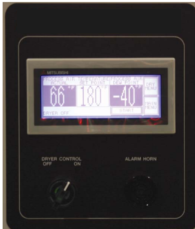
Figure 3: Typical Control Panel
