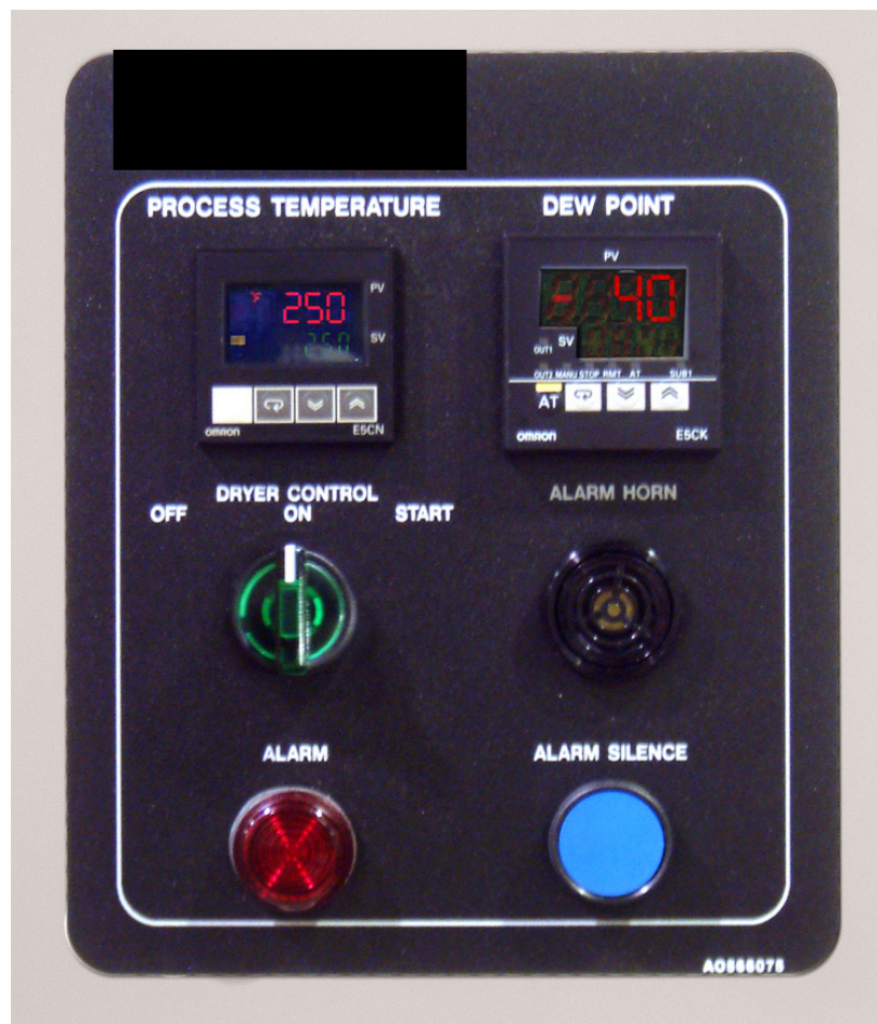
Figure 4: Typical Dryer Control Panel
