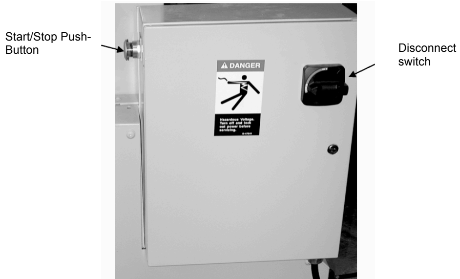
Figure: Control Panel
