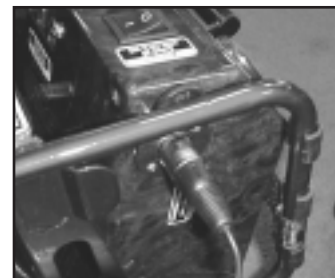
Off-board charger port
