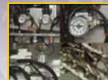
Temporary monitor of plumbing and pump pressure such as in air conditioning repair
