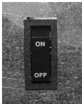
Figure 15: Blower fan switch.
