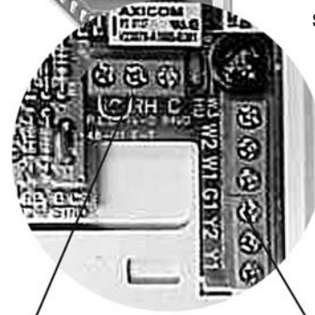
Figure 7: Wiring the DEH 2000 control.
