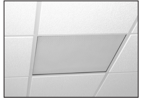
Fig. 10: Completed subwoofer installation.
