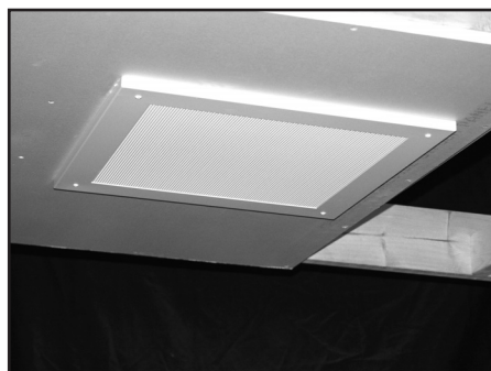
Fig. 10: Completed subwoofer installation.
