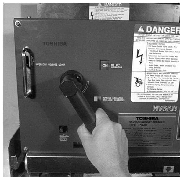
Fig. 26 Manually Charging Breaker
