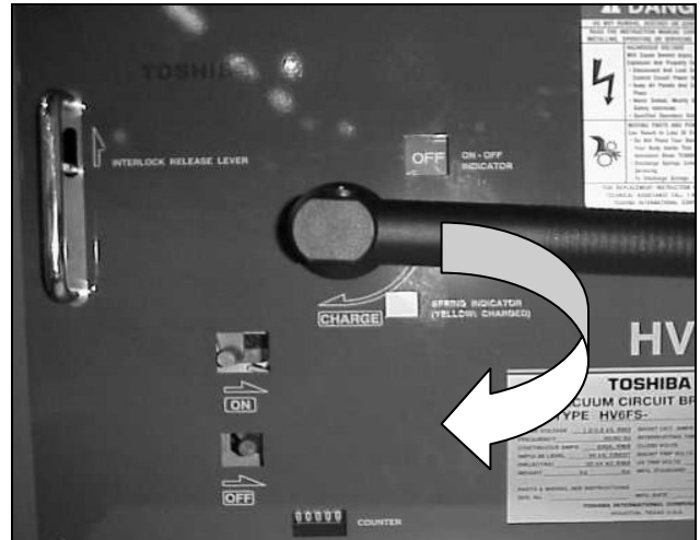
Fig. 25 Preparing to Manually Close Breaker
