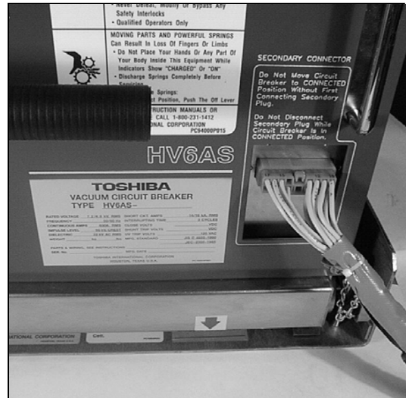
Fig. 21 Control Circuit Plug Connected to Breaker
