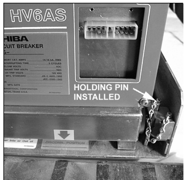
Fig. 20 Breaker at DISCONNECTED Position
