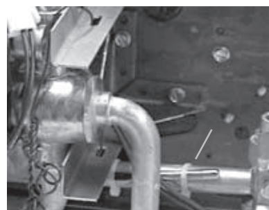
Figure 14. The changeover sensor strapped to the supply water pipe.
