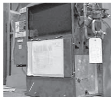
Figure 22. Locate the wiring schematic on the fan and motor panel of vertical concealed and all horizontal units. (This unit is turned on its side.)
