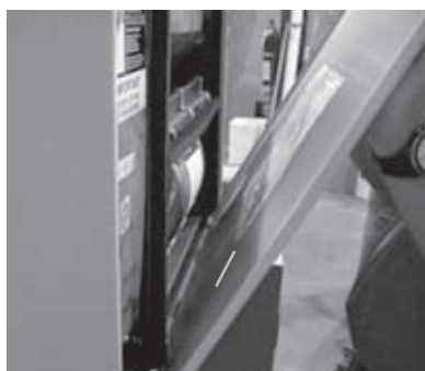
Figure 21. Locate the wiring schematic on the inside of the front panel of vertical cabinet and recessed units.
