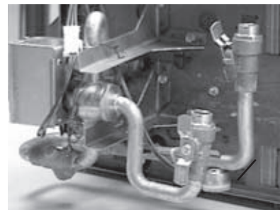
Figure 15. Units with electric heat have an electric heat lockout switch on the supply water pipe.
