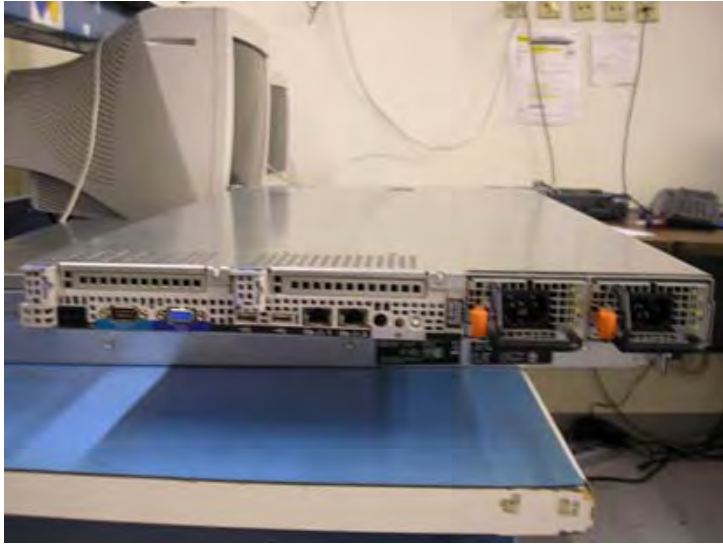
Figure 1. VOD 50W (Dell 1950 – Rear View)
