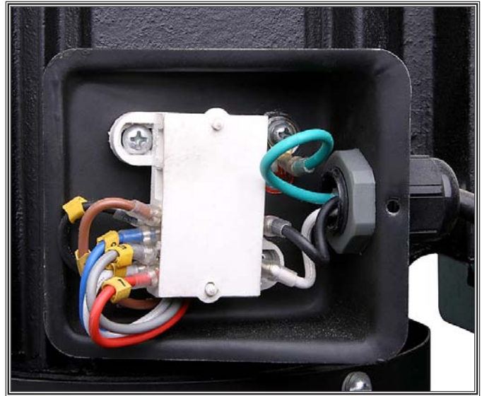
Figure 35. Motor junction box wiring.
