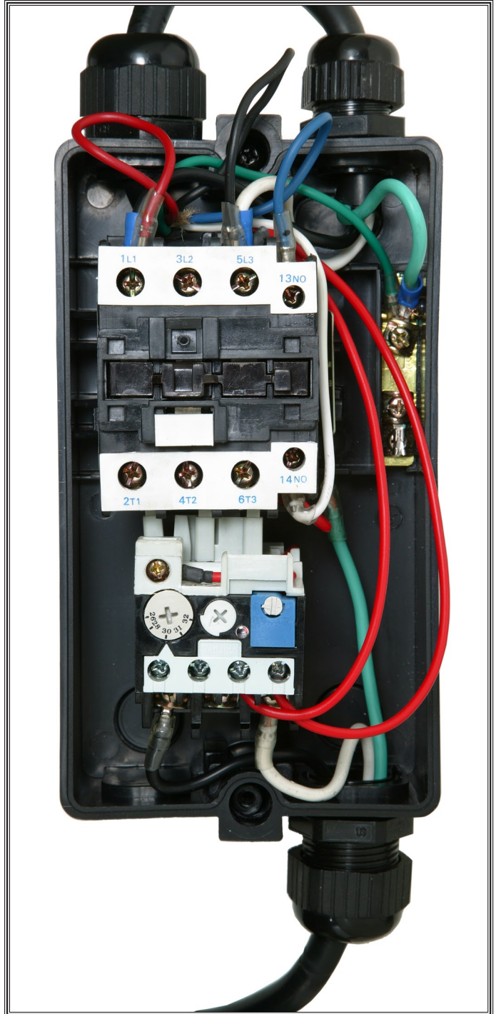
Figure 43. W1754 magnetic switch assembly.
