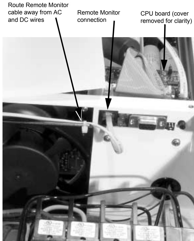
Figure 2-18 Remote Monitor connection and cable
