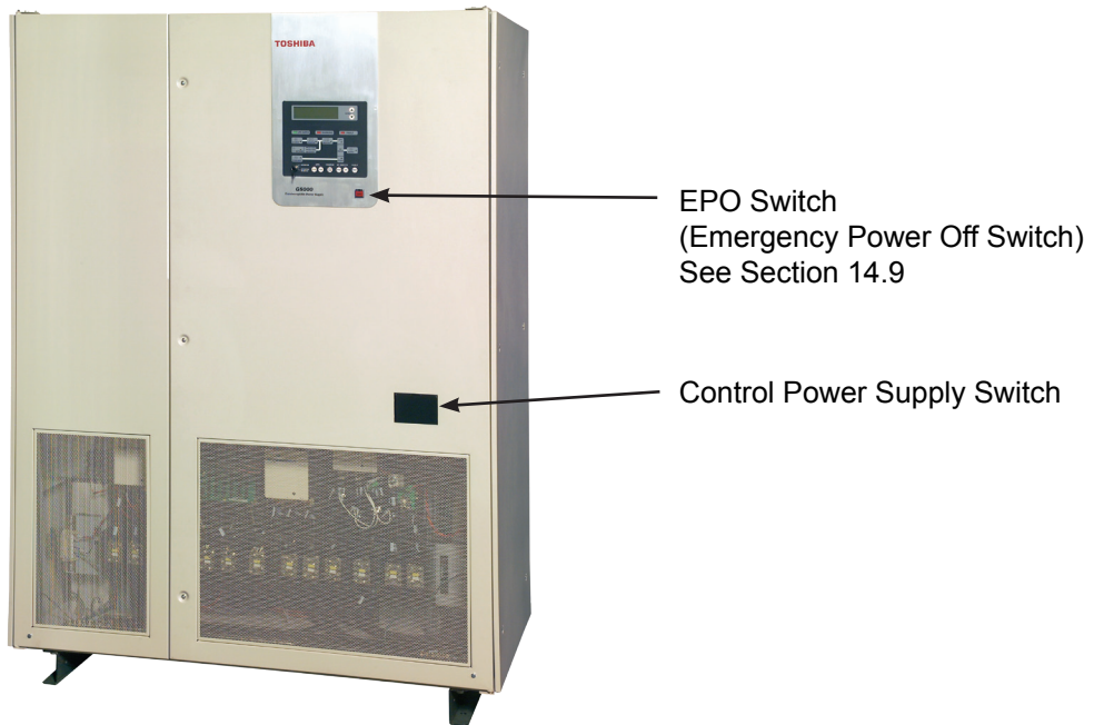
FIGURE 14.1 - EPO AND CONTROL POWER SUPPLY OPERATING SWITCHES
