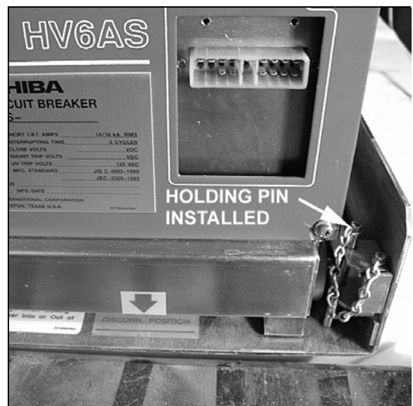
Fig. 20 Breaker at DISCONNECTED Position
