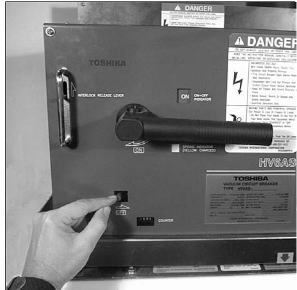
Fig. 27 Manually Opening Breaker
