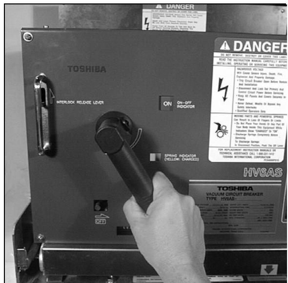
Fig. 26 Manually Charging Breaker
