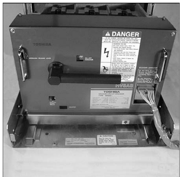
Fig. 22 Breaker at CONNECTED Position
