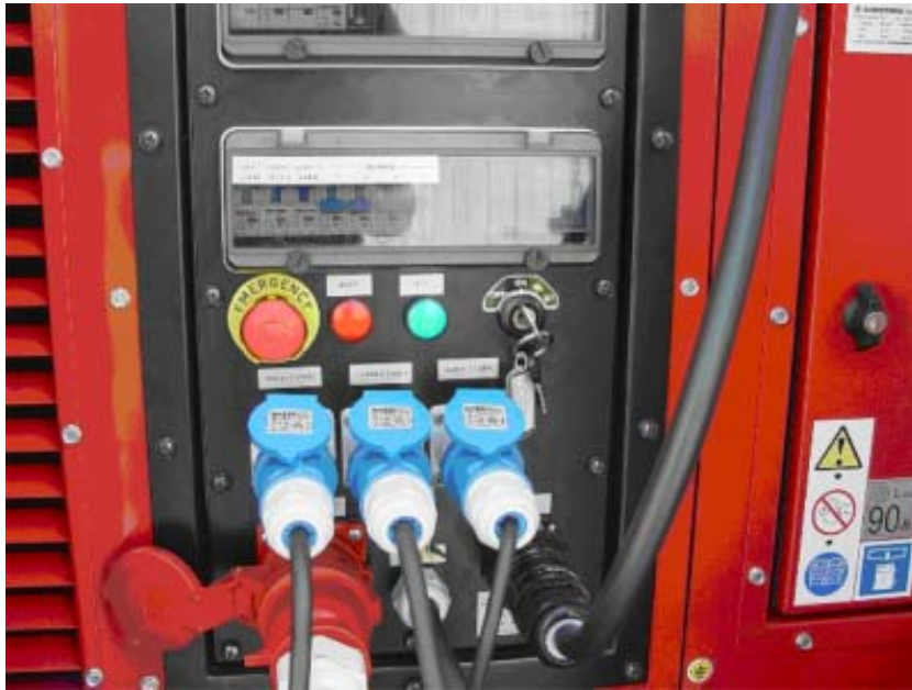
Image 2-8 Control panel generator
