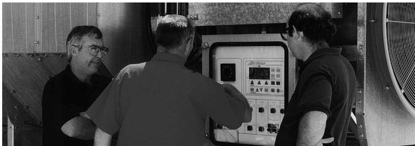
Dryer owner and Airstream associates check the Electronic Monitoring Control System.
