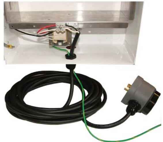
Fig. 4-4, Streetlight AC Power Tap Cable Installed
