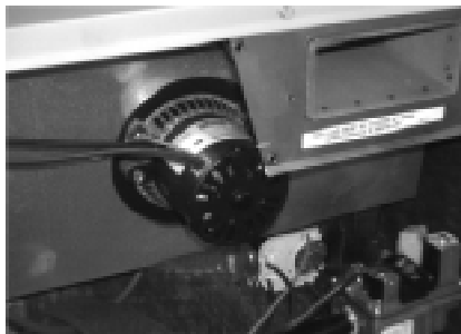
Figure 22 Induced Draft Motor
