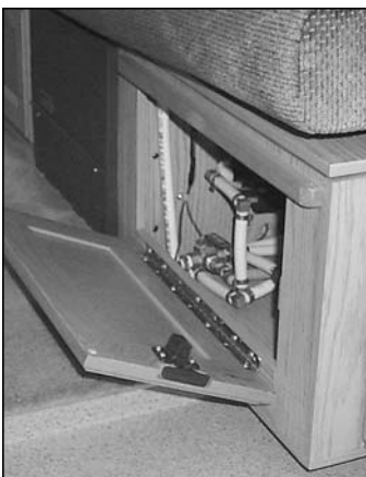
Picture G-P16: Location of the access door for the tank selector valve.
