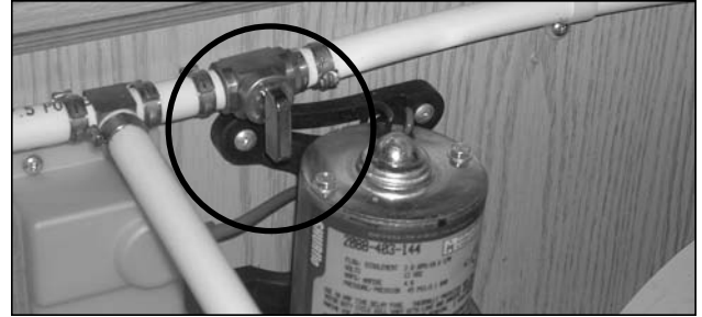
Picture G-P20: Hot water cutoff valve in closed position.
