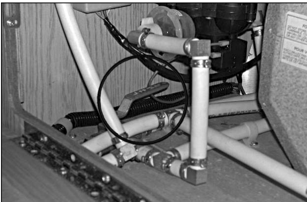
Picture G-P12: Selector valve supply from the exterior fresh water tank.
