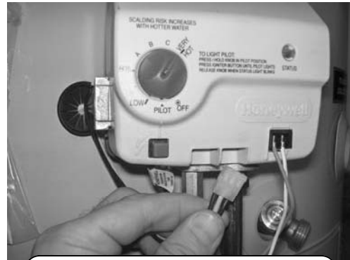
Wire harness plug in location to the gas control
