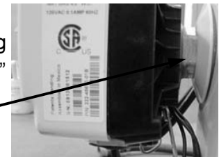
Flats of thermal well
