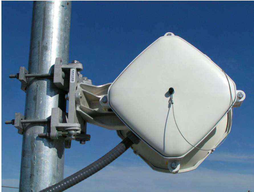
Figure 3-11: Back view of fiber and power cable installed on a vertically polarized unit. Notice that the cable conduit is on the left hand side when the radio is in (V) polarization.
