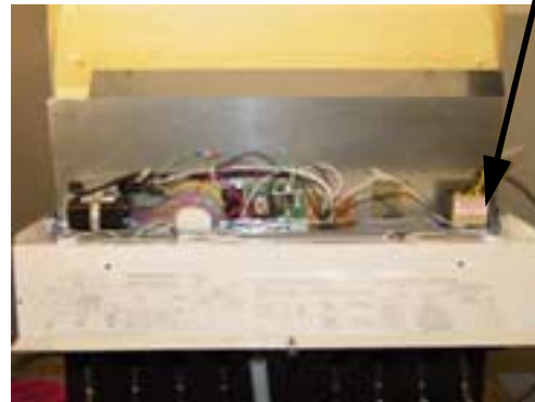
FIGURE 29. Electrical Box 2x Single Transformer
