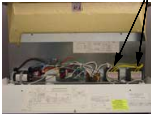
FIGURE 30. Electrical Box 2XX Dual Transformer
