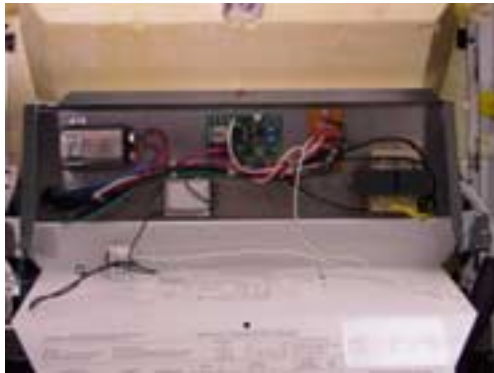
FIGURE 28. Electrical Box 1x Single Transformer
