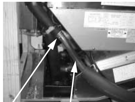
Clamp Drain Line
