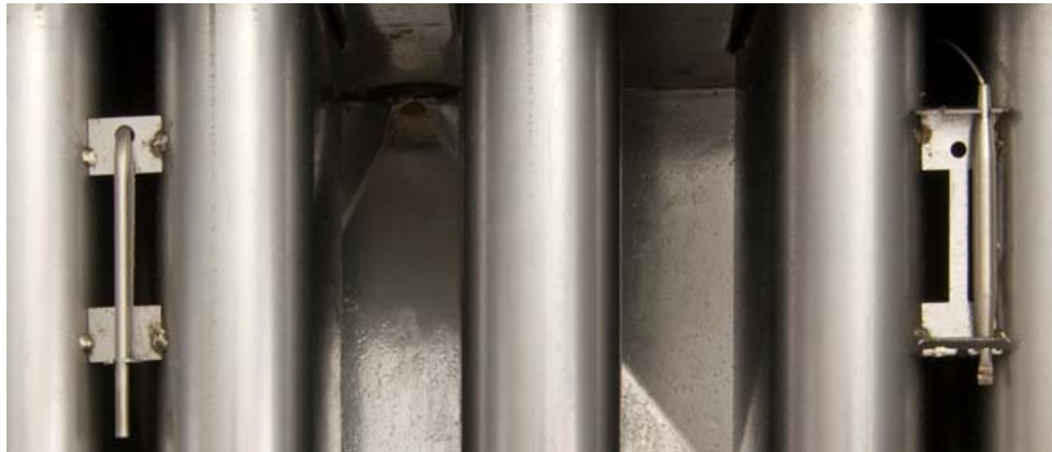
Typical sensor probe/high-limit locations and mounting hardware.
