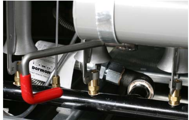
A microswitch is located on the red handle at the drain valve.
