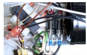
Transformer and fuses.
