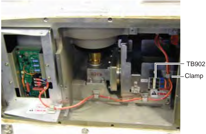
Antenna unit, cover removed (left-hand side)
