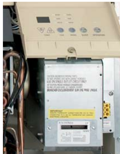
Enclosure cover removed.
