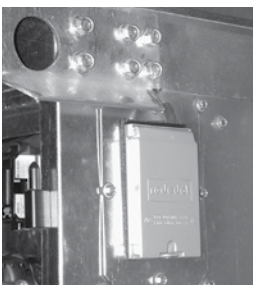
Manual High Voltage On/Off Switch with Lockout
