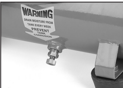
Figure 10. Tank drain valve.
