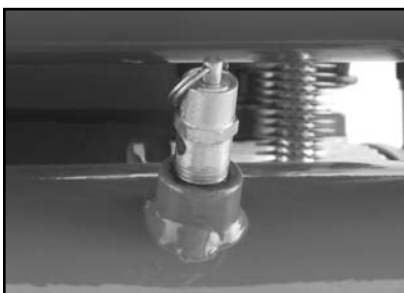
Figure 8. Safety drain valve.
