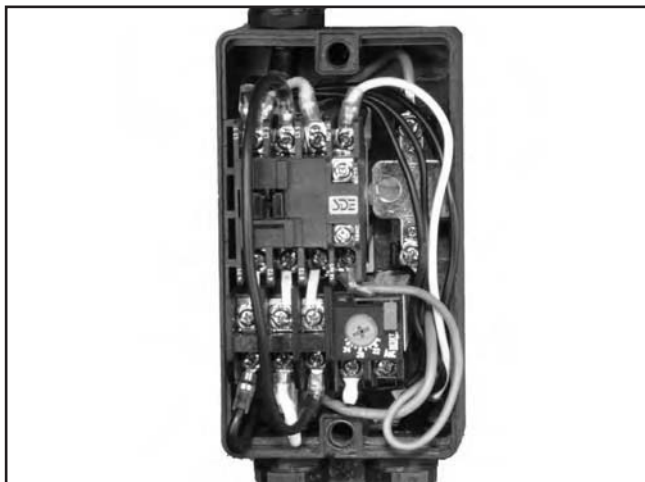
Figure 4. 220V Magnetic Switch
