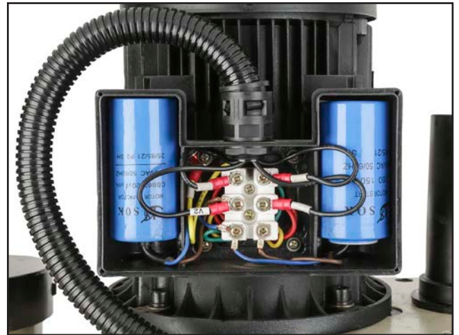
Figure 48. Motor junction box wiring.
