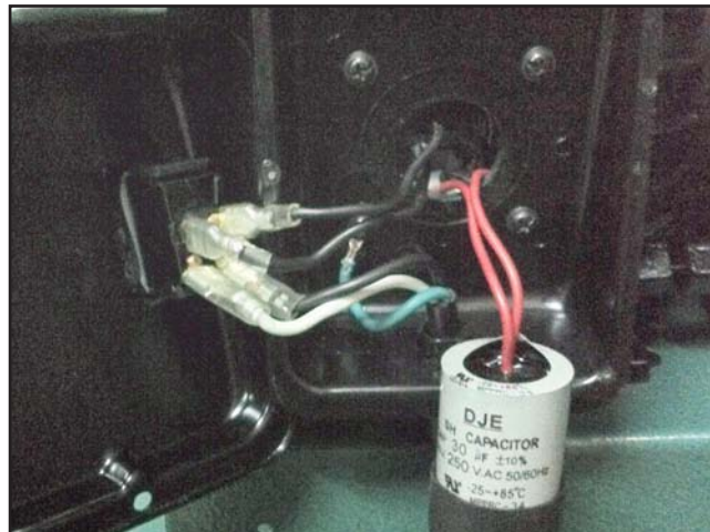
Figure 71. G0548Z junction box, switch and run capacitor.
