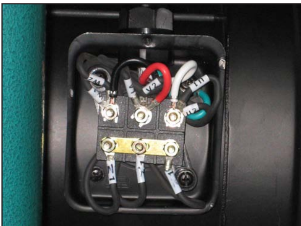
Figure 157. G0606X1/G0697X motor junction box.
