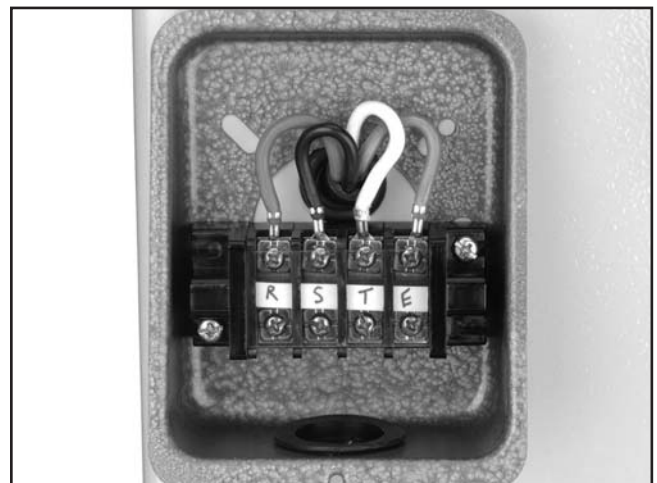
Figure 29. Main terminal located inside the electrical wiring box, on the outside of the cabinet.
