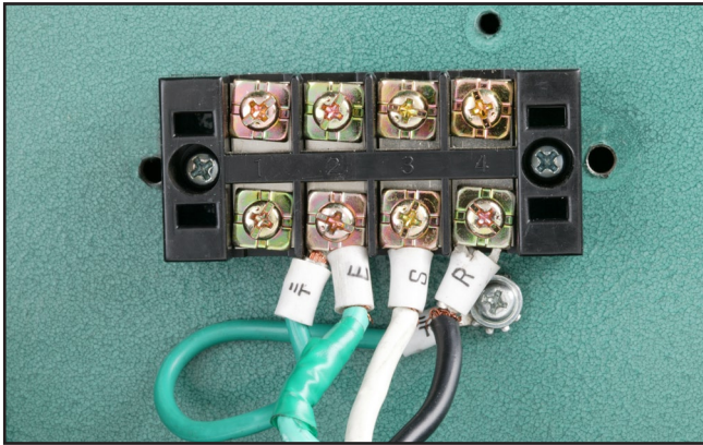
Figure 70. Power supply terminal box.
